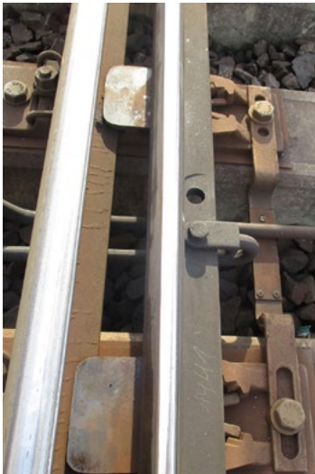
Open switch rail
